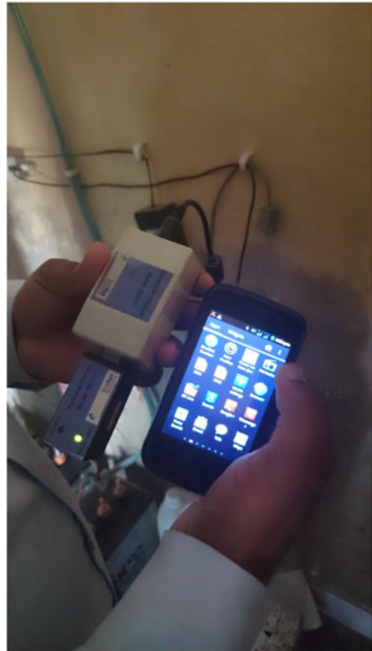
Figure 3. The pre-payment dongle of a pico-grid for charging the solar credits.
